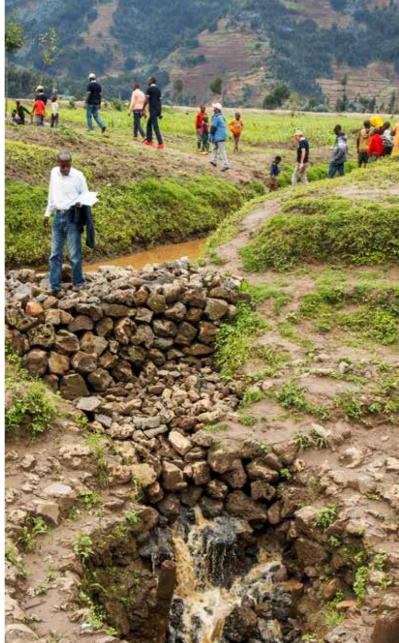
A stormwater drainage project in a flood-prone valley in the north-west volcanic region of Rwanda.
